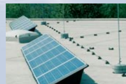
Lightning Protection / Earthing
